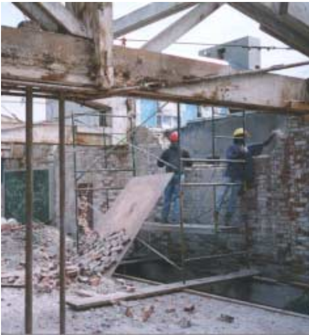
Salvaging bricks from a Vancouver warehouse. Mortar is removed on site and bricks are packaged on pallets of approx. 500 units. Broken and damaged bricks are recycled.
